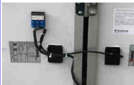
Back of Solar Panel Connections
